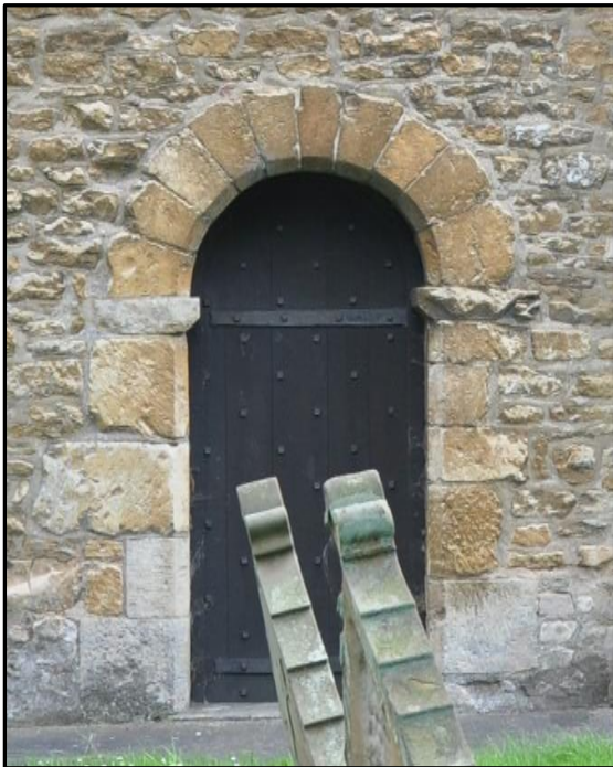
Further thought considered that the sophisticated chamfered edges placed the architecture of the doorway in the Norman period.
