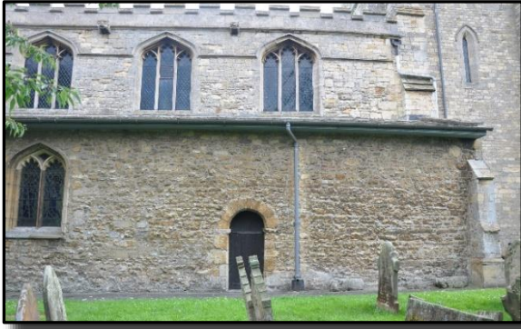
During refurbishment in 1929 the doorway (seen centrally above) was re-discovered and originally thought to be Saxon.
