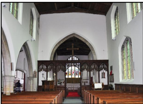
Inside the church, the chancel arch is C13 Early English whereas the windows are C15 perpendicular style as is the nave roof.
