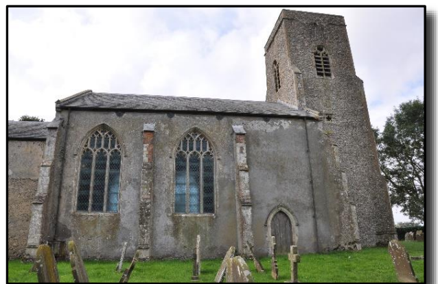
Looking at the base of the east window from inside the church reveals that the window's source was . . .
