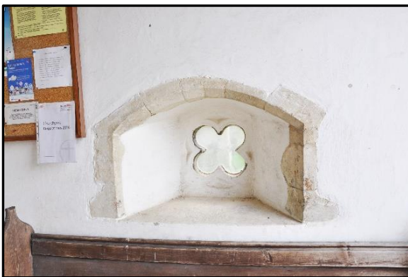
These attractive and unusual features are set into embrasures in the porch walls.
