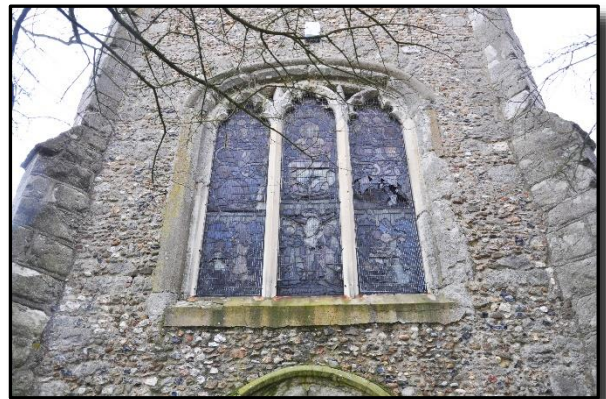
This might indeed be correct - but the western window (seen above) is in poor condition and there seems to be no evidence of change in the supporting stonework.
