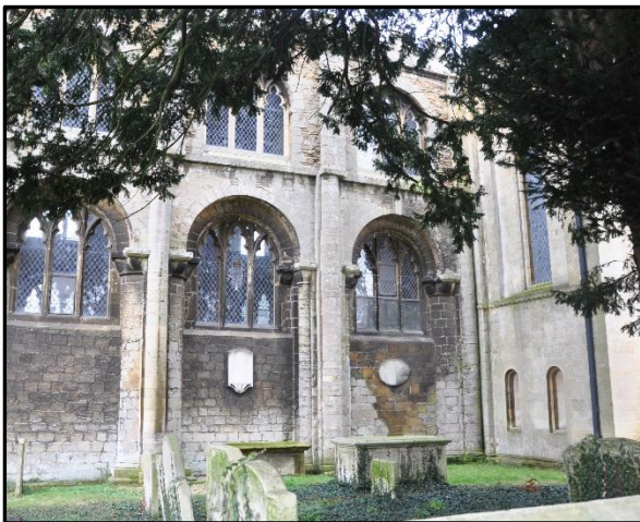
This picture shows the transition of the stone type from the rough C12 ashlars of the wall of the nave to the smoother ashlars of the C19 wall of the transept.
