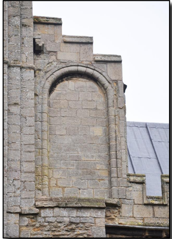
Adjacent to the sundial is a blocked up Norman-arched doorway. There is a similar one below it.
