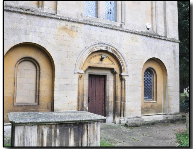
Here you see the south wall of the C19 transept where it is clear that the stonework is vastly different.
