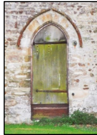
From the outside one can see the repeat of the two-centred round arch visible inside. This suggests that, rather than this originally being a Saxon doorway to which the round arch has been added, it is the inverted-V lintel which has been added inside (perhaps in C15?) to support the C13 arch.
