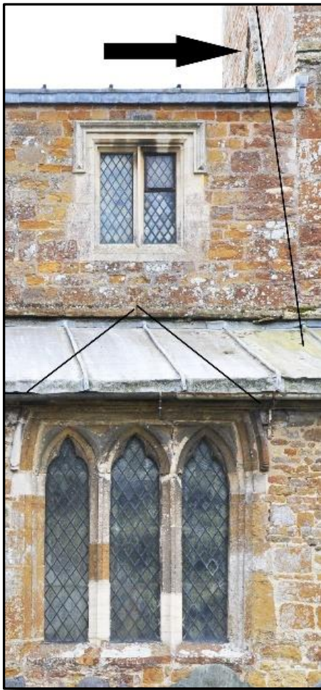
Looking at the west wall of the tower we can see signs that there was originally a steeply-pitched roof here which was removed when the clerestory (with the square-framed windows) was added in c.1470. The earlier roof would have followed the drawn line downwards. The other two lines indicate the former profile of the three-light lower window before it was cut short by the new lower roof.
