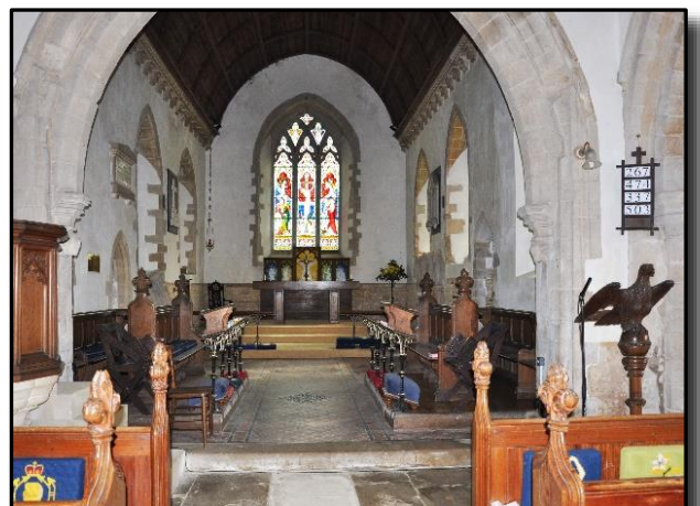
The chancel and chancel arch. The latter has areas of damaged stone which indicate the original position of a rood screen.
