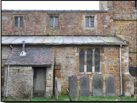
The north wall looks a little gloomy with its C20 addition of a boiler house but it seems it did not always look this way.
