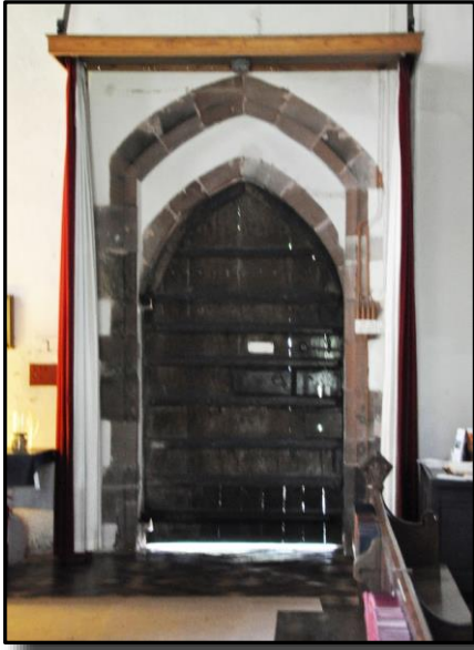
The masonry arch over the south doorway is the oldest piece of fabric in the church the rest of the nave having been rebuilt in C14. This arch remnant dates from C12.
