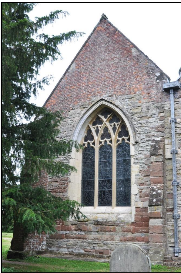
The west wall of the north aisle has, at the top, been repaired with red brick. The records suggest that this would have been carried out in C17 at the same time that the east end of the church was restored.
