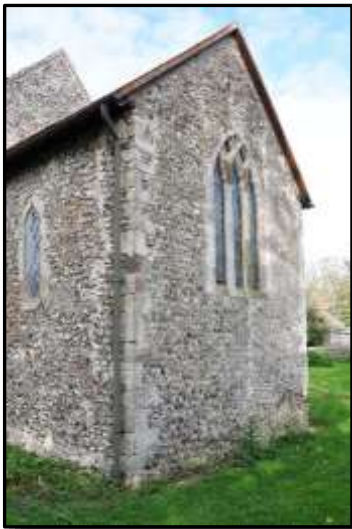
The quoins used as corner stones are quite massive and records tell us that many of them have been repositioned.
