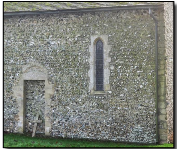
This is the western half of north wall showing the blocked north doorway
